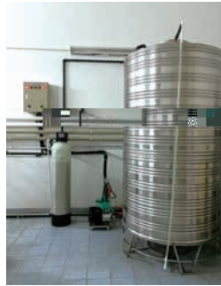
Drinking water recycling system (Shenzhen facility)
